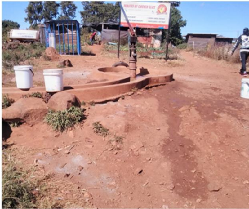
Borehole and LP Gas outlet
